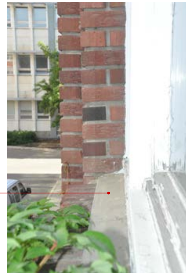
Figure 34 - 1946 Window Exterior Sill Condition
