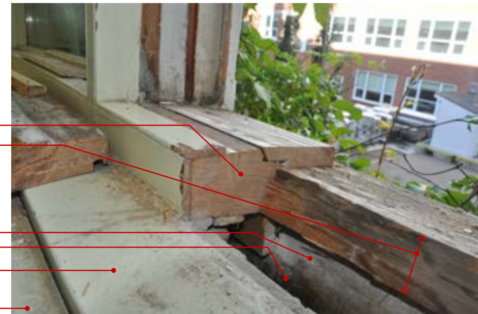
Figure 19 - 1922 Window - Level 2 Sill
