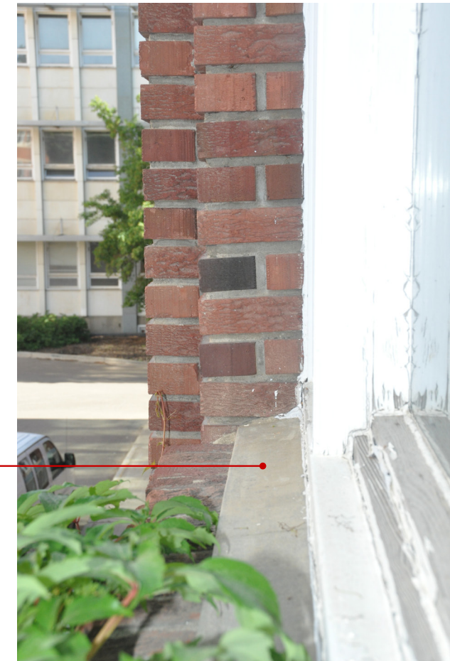
Figure 34 - 1946 Window Exterior Sill Condition
