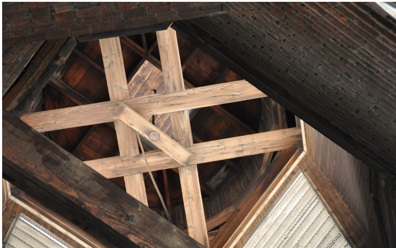
Figure 53: 1922 Spire Interior - Black stains indicate mold growth on wood members.
