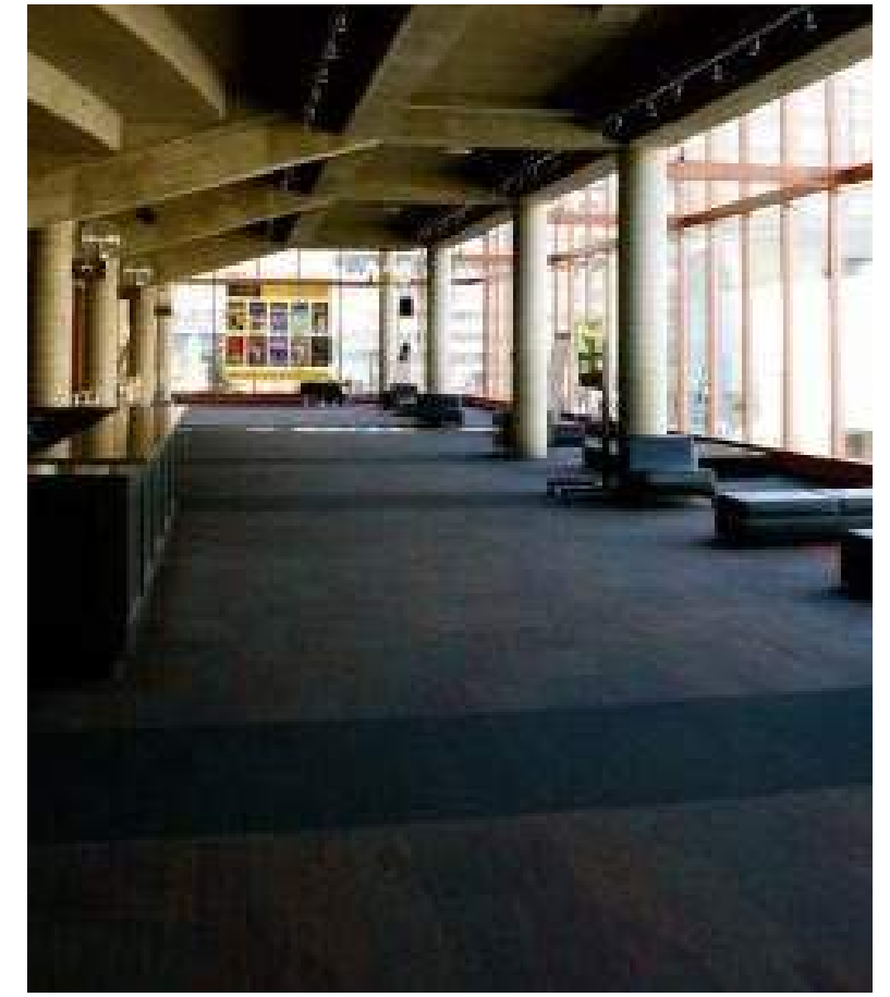
Charcoal carpet tile is a maintenance friendly alternative to replace the deficient broadloom that currently exists in the space.
