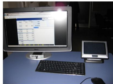
AMX control panel and touchscreen display.
